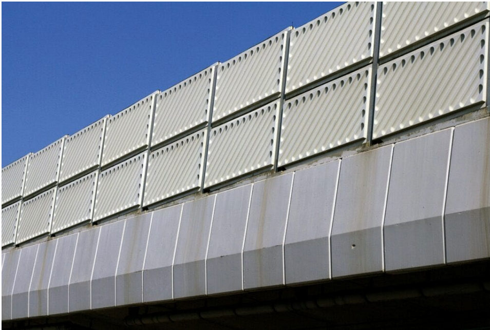
Figure 19. Tyre-based noise walls (Roadline, 2022).
